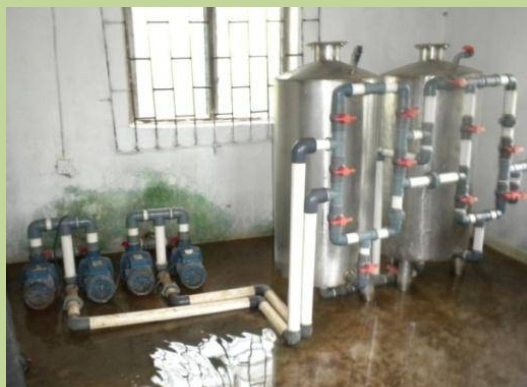
Expensive, complex and difficult to operate and maintain water treatment system at Olougbene in Egbema-Gbaramatu RDC
